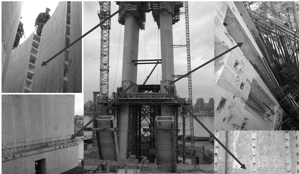
Slika 6. Primena mehaničkih spojnika – Most preko Ade u Beogradu Figure 6. Rebar Couplers Application – Ada Bridge in Belgrade
