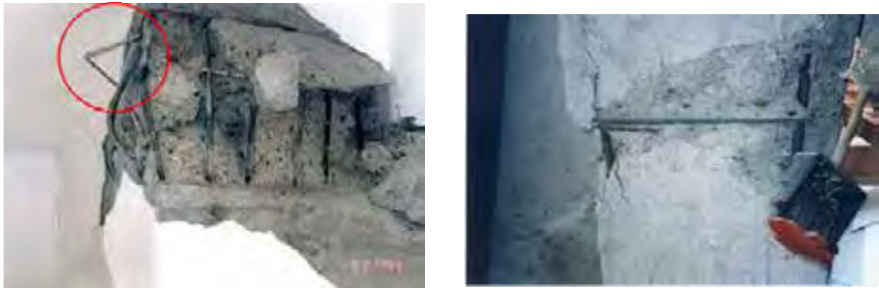
Fig. 34. Initiation of column failure due to 90° hooks of stirrups – Turkey 1999
