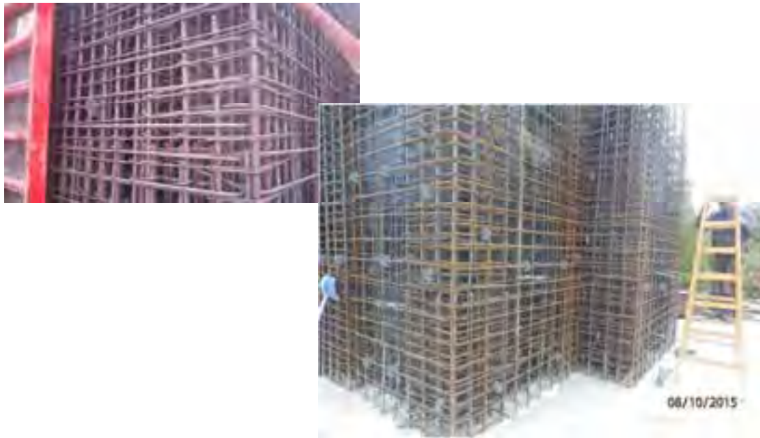
Fig. 22. The confining reinforcement of wall with composite section designed according to Eurocode 8 (note the example building presented on Fig. 6 and Fig.7)
