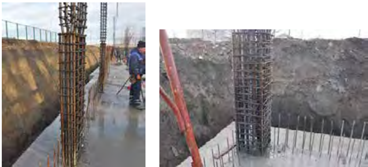
Fig. 35. Problems with clear space between both longitudinal and transverse reinforcement in lapping length of longitudinal bars (the structure was designed according to Eurocodes)
