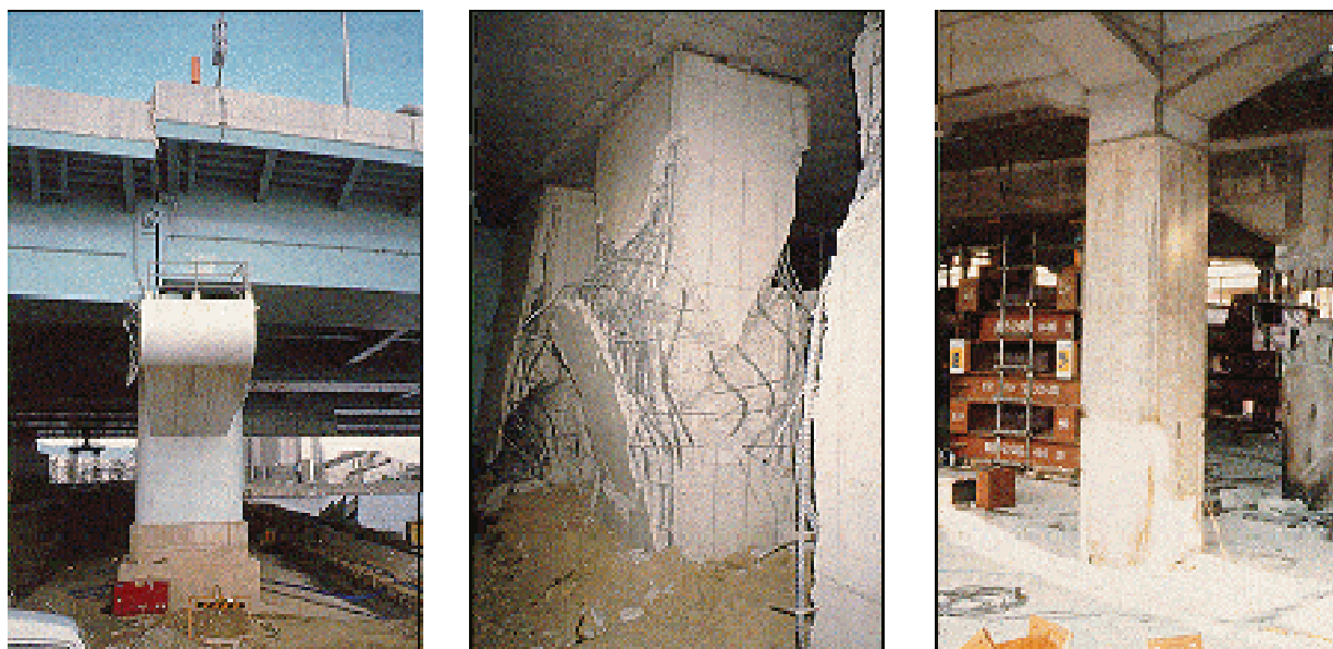
Figure 1. Shear failure of piers of the Hanshin Expressway in Kobe during the Hanshin-Awaji earthquake (from www.fhwa.dot.gov )
