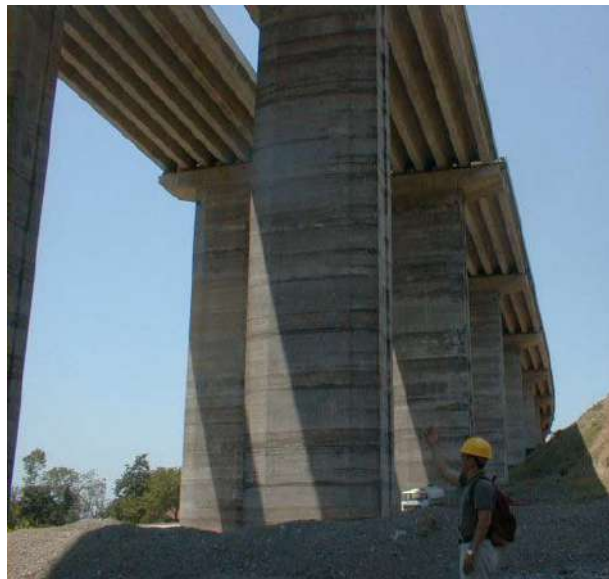
Figure 10. Bolu viaduct with large permanent offset due to fault rupture (from www.purdue.edu )
