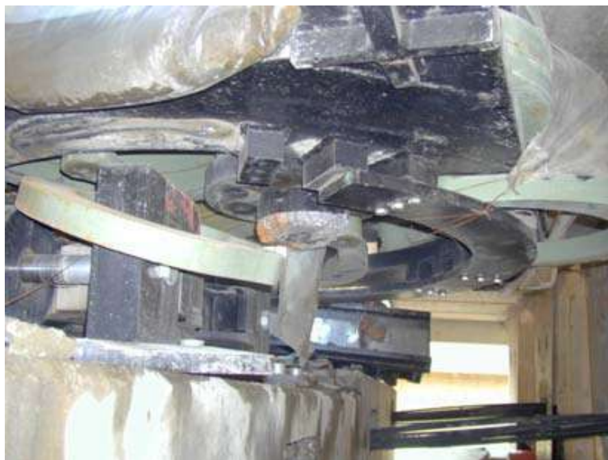
Figure 11. Over-extended "moon shaped" elastic plastic device in the Bolu viaduct [11] due to permanent fault line displacement. These devices were replaced by LRBs
