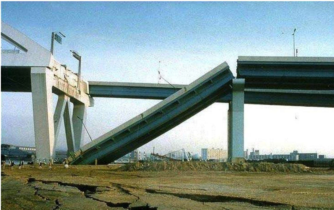
Figure 2. Drop-off of a large steel section of the Hanshin Expressway during the Hanshin-Awaji earthquake (from www.washington.edu )
